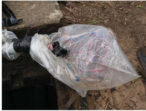
“Temporary” repairs. Note condensation inside bag.
